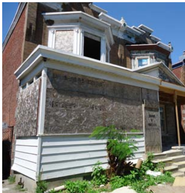
Bottom: One of 30 single family homes in Camden’s Parkside neighborhood that has since been rehabilitated using NRTC dollars.
